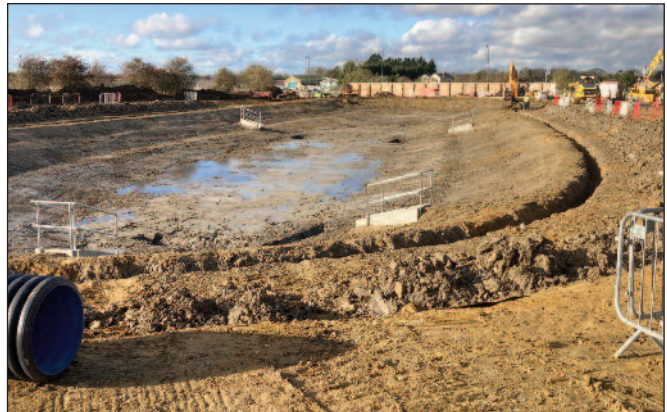
POND-DIPPING: A new attenuation pond takes shape to replace the existing one.
